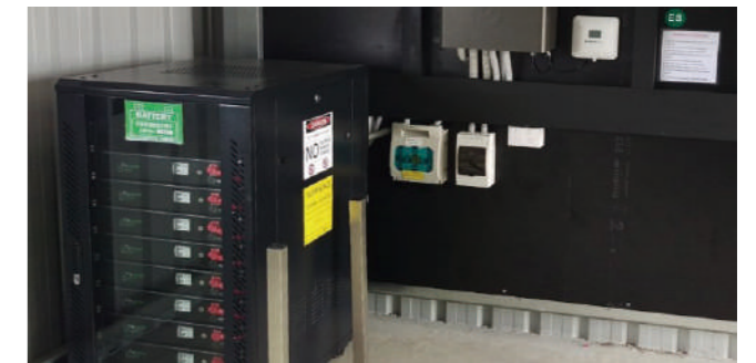
Rack-mounted lithium battery
